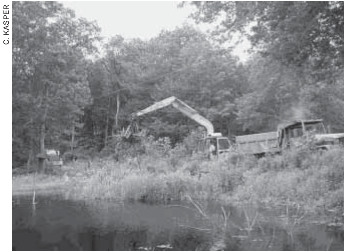
Beaver debris was removed from water control structures at 10 state impoundments.
