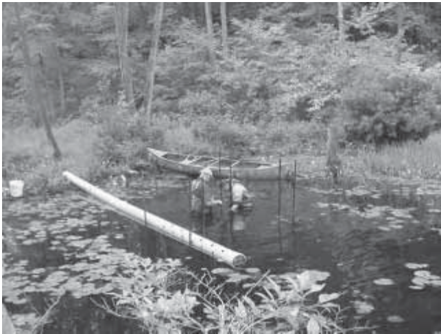
Piping and fencing were installed at 10 marshes in an effort to restore lower water levels for wildlife use.
