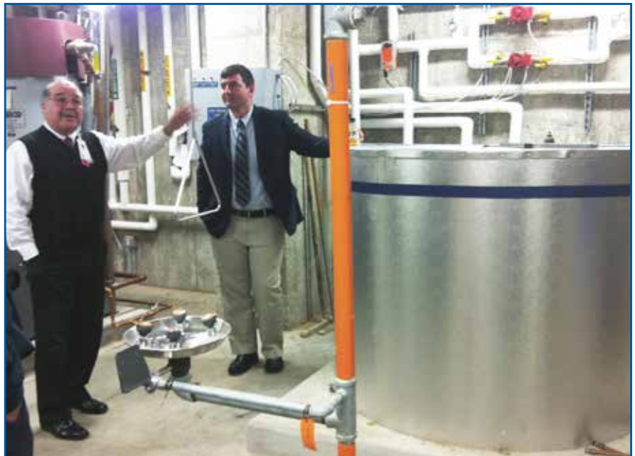
Mark Vere of Gaylord Hospital and Orlin Karabadzhev of Legacy Mechanical Group at the storage tank discussing the solar thermal distribution system.
