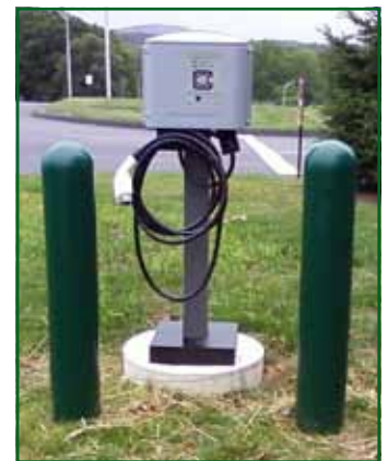
Vehicle charging station
