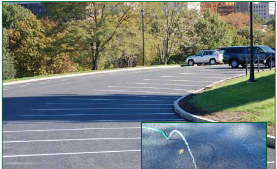
Porous asphalt at the State Capitol parking area. Right: Demonstration of absorption capacity.
