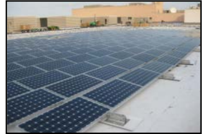
Figure 2 Solar PV array installed on the roof of the Atlantic City Convention Center by Pepco Energy
